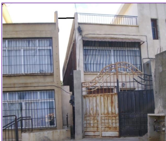
Figure 6 : Écartement du joint de dilatation. Figure 6: Spacing of the expansion joint.
